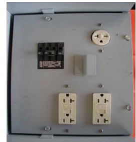
Figure 12. Non-metered Temporary Service Panel
