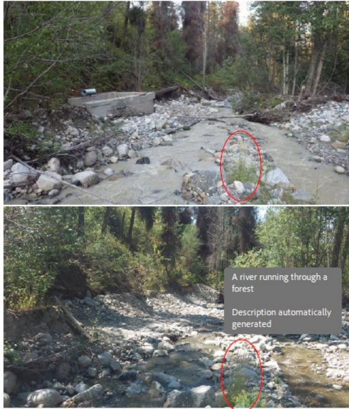
Figure 3 Top: Preconstruction photo of diversion infrastructure August 6 th , 2024. Bottom: Postconstruction photo of diversion infrastructure site looking downstream at re graded left bank August 7 th , 2024. An undisturbed patch of grass is highlighted as a reference point in both photos.
