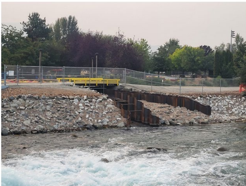
Looking towards east bank (river left) at south end of fishway with vehicle bridge
