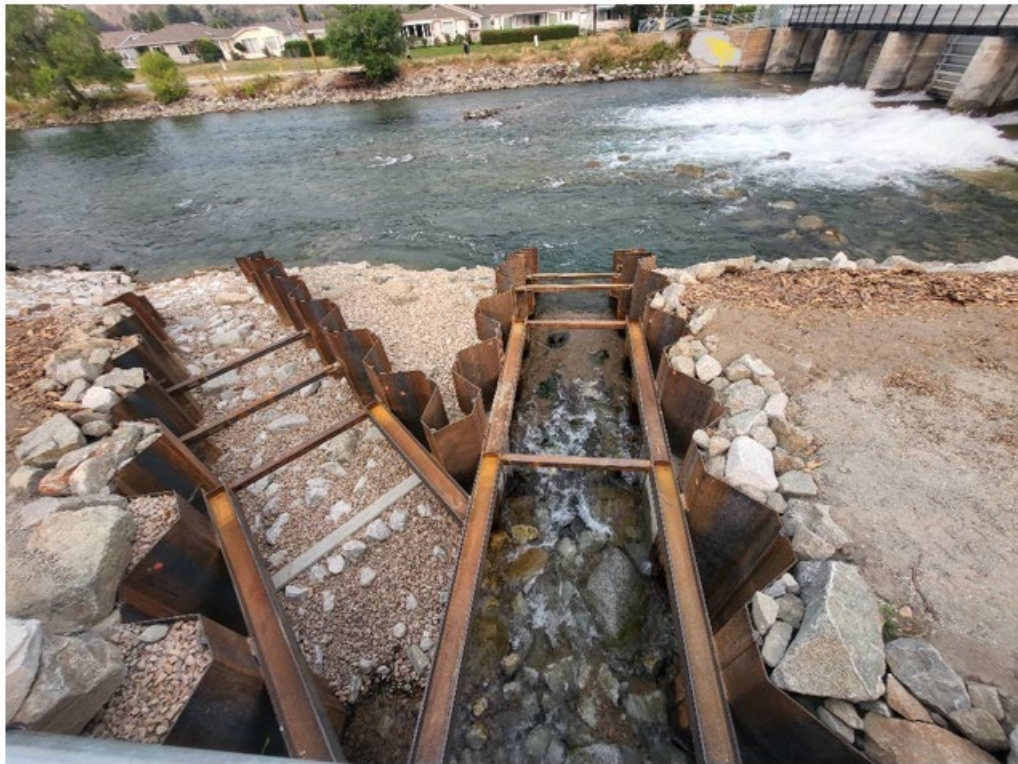
South end of fishway with high and low flow fish entrance channels
