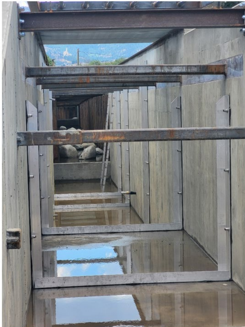
Stop log guides installed at north end
