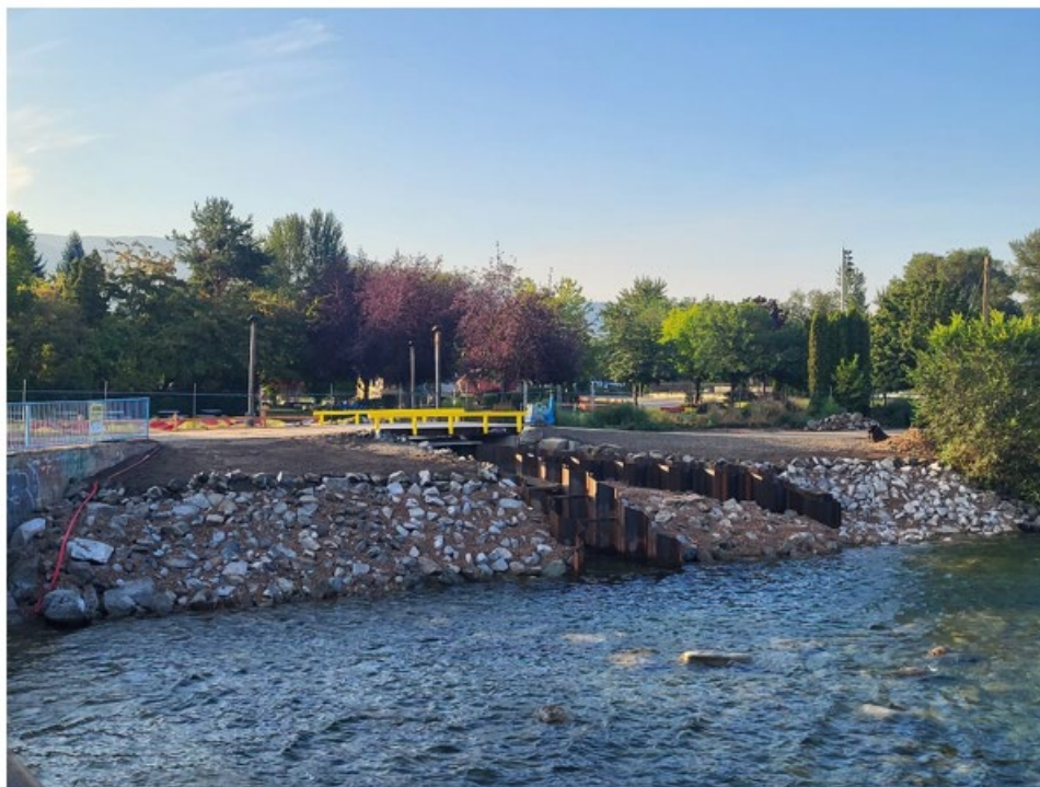
South end of fishway with high and low flow fish entrance channels
