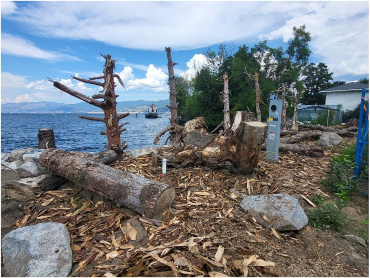
Mulch added to protect soil for fall planting. Electrical pedestal in place.
