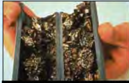
Zebra mussels in a out-away pipe
