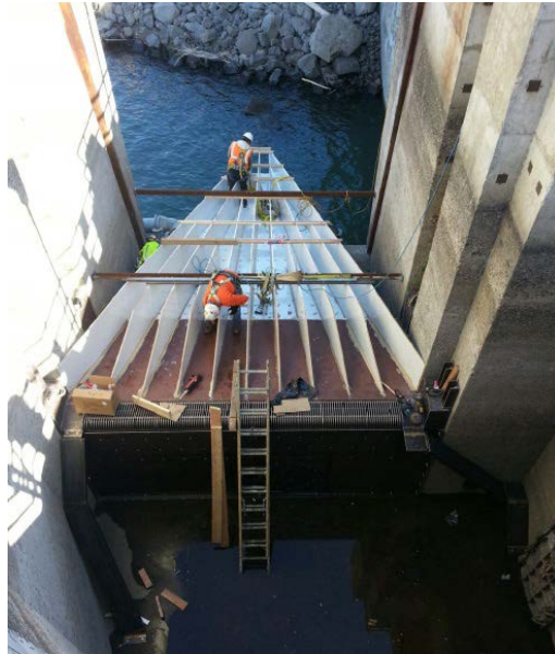
Figure 1 Construction activities related to the installation of the Wanapum Left Bank Fishway Exit Passage System.
