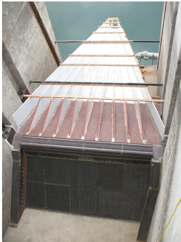
Figure 4 Wanapum Right Bank Fishway Exit Passage System. Completed and operational on April 26, 2014.
