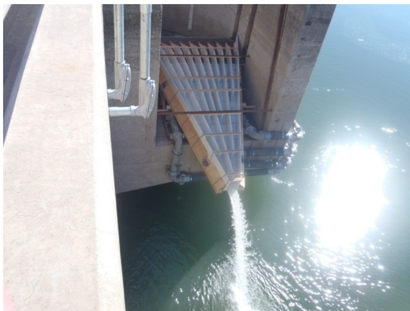
Figure 2 Wanapum Left Bank Fishway Exit Passage System – Flume.
