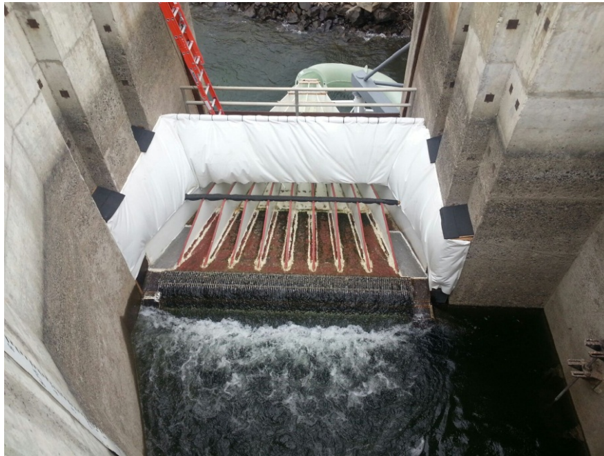
Figure 3 Photograph of jump curtain installed at the Left Bank Wanapum Fishway Exit Passage System and the system in operation.
