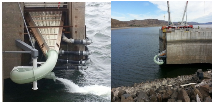
Figure 1 Photograph of installed spiral chutes at the Left Bank and Right Bank Wanapum Fishway Exit Passage System. The spiral chutes were installed on the left and right bank fishway exit passage systems on June 12 and June 19, 2014, respectively.
