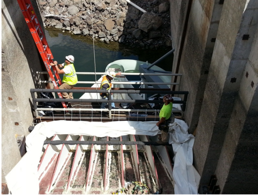
Figure 2 Photograph of installation of jump curtain at the Left Bank Wanapum Fishway Exit Passage System.
