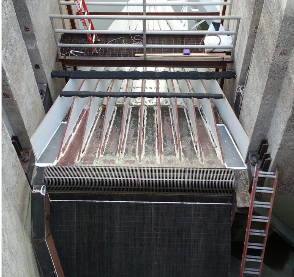
Figure 5 Perforated plating added to the false weir floor and vane walls to preclude adult lamprey from re-ascending and reentering false weir pool. The perforated plating was installed on June, 12 (left bank) and June 19 (right bank), 2014.
