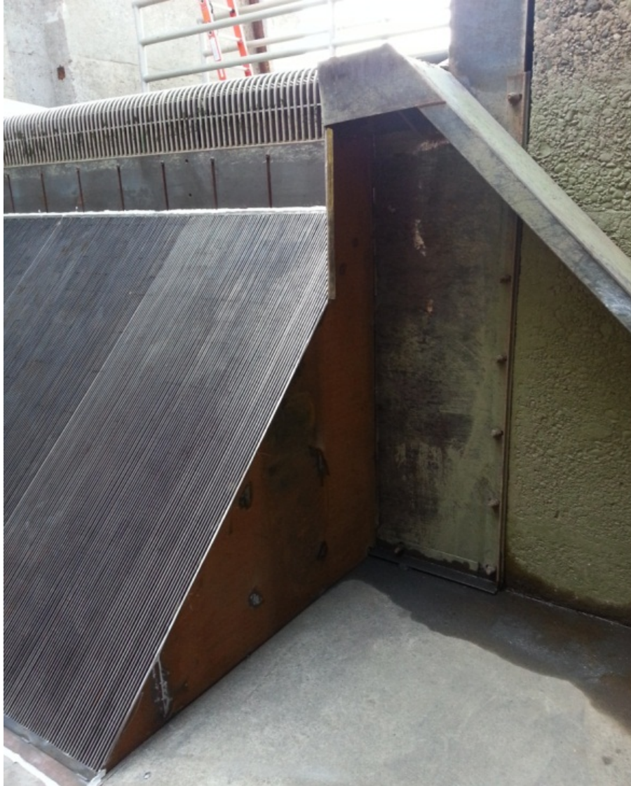
Figure 4 Approach ramp/anti jump ramp and lamprey ramp (upper right hand corner) installed at the Left bank Wanapum Fishway Exit Passage System. The approach ramp/anti jump ramp was installed on June, 12, 2014.
