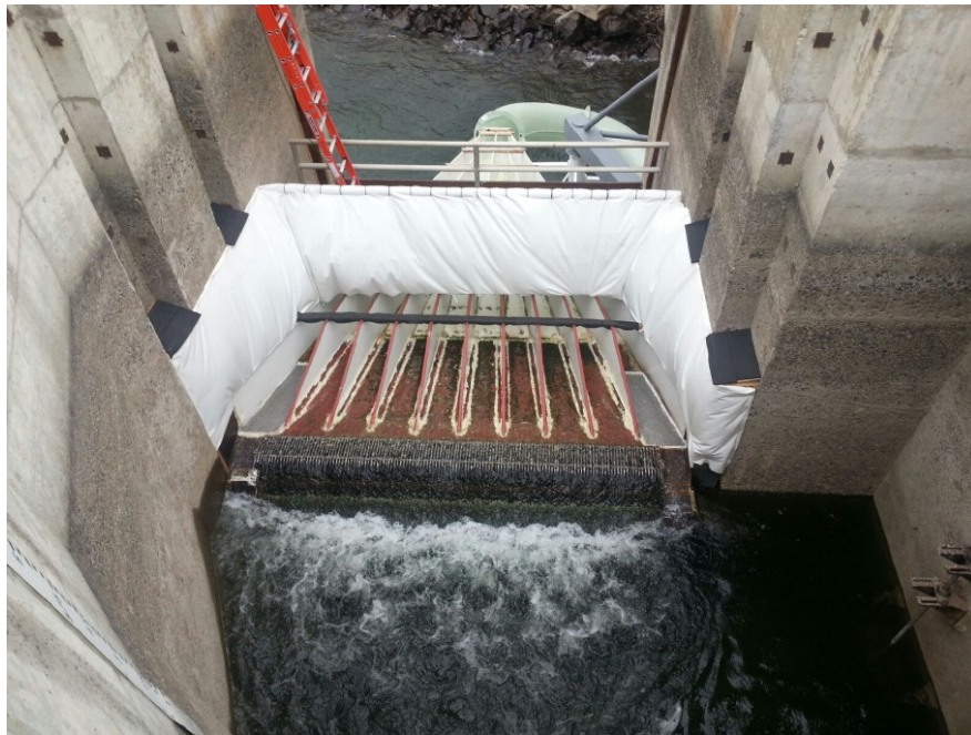
Figure 2 Photograph of jump curtain installed at the Left Bank Wanapum Fishway Exit Passage System and the system in operation.
