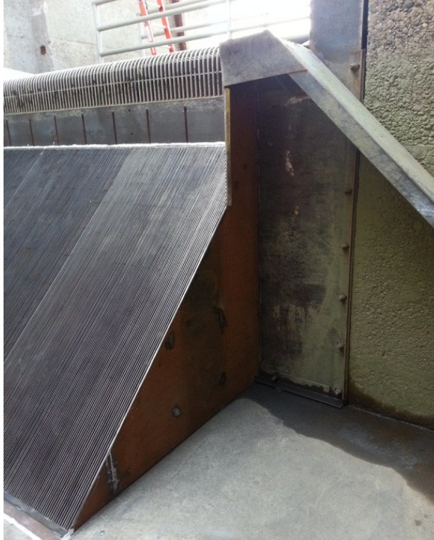
Figure 3 Photograph of approach ramp/anti-jump ramp and lamprey ramp (upper right hand corner) installed at the Left Bank Wanapum Fishway Exit Passage System. The approach ramp/anti-jump ramp was installed on June 12, 2014.
