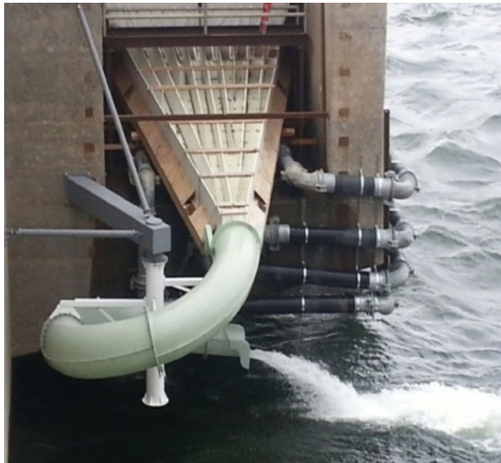
Figure 4 Photograph of installed spiral chute at the Left Bank Wanapum Fishway Exit Passage System. The spiral chutes were installed on the left and right bank fishway exit passage systems on June 12 and June 19, 2014 respectively.
