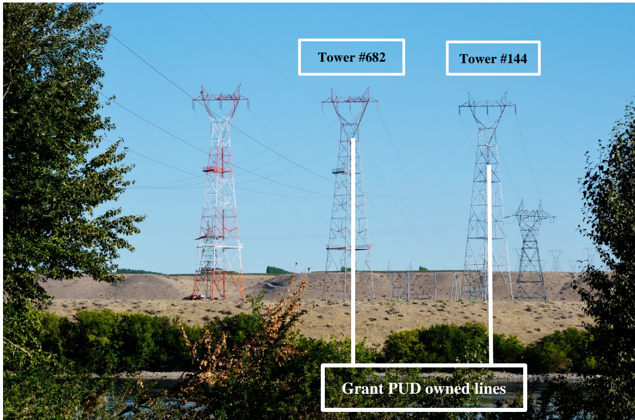
Figure 3 The three-span transmission line cluster at Midway with Midway – Frenchman Hills 230kV line between Structures #681 and #682 and Priest Rapids – Midway 230kV Line #2 between Structures #144 and #145 identified.
