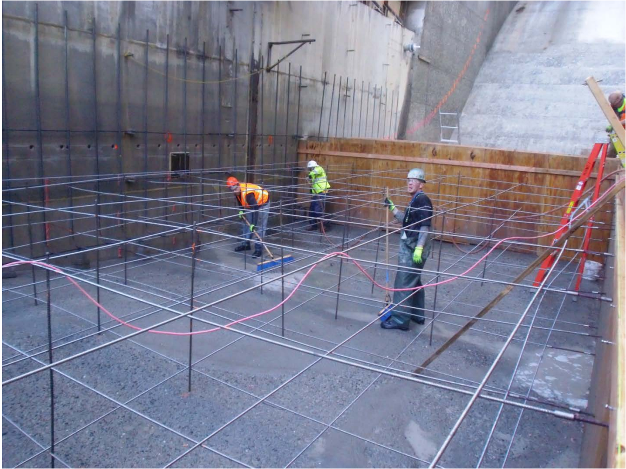
Figure 6 Priest Rapids Fish Bypass – Spill bay 22 mass concrete form work – apron pour.
