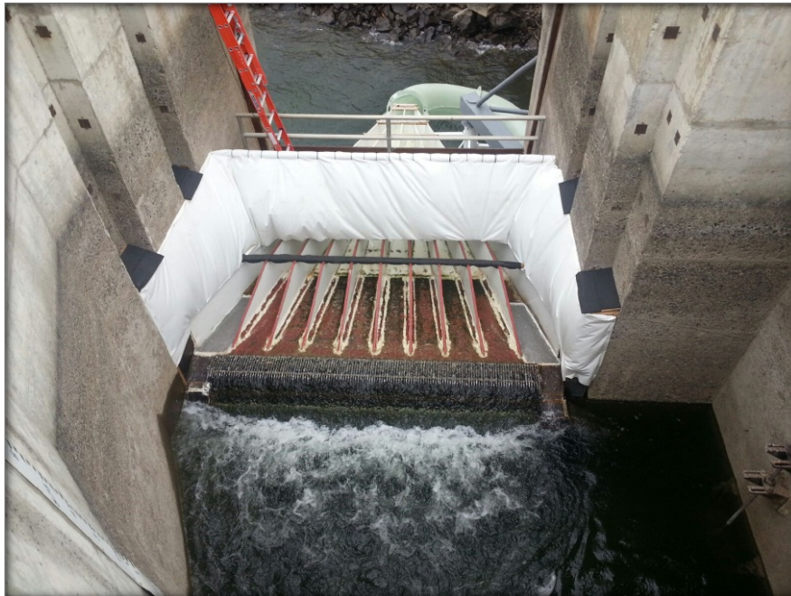
Figure 9 Photograph of jump curtain installed at the Left Bank Wanapum Fishway Exit Passage System and the system in operation.
