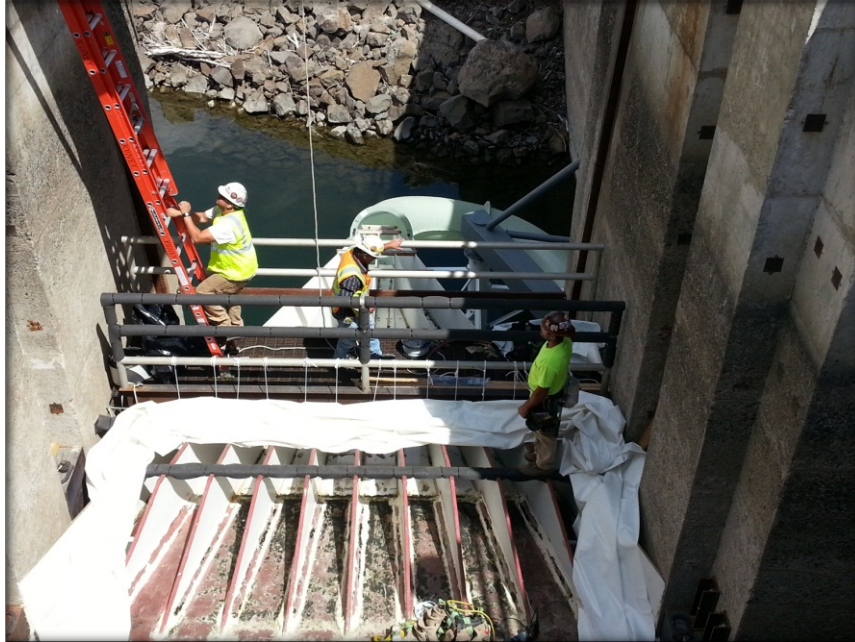
Figure 8 Photograph of installation of jump curtain at the Left Bank Wanapum Fishway Exit Passage System.
