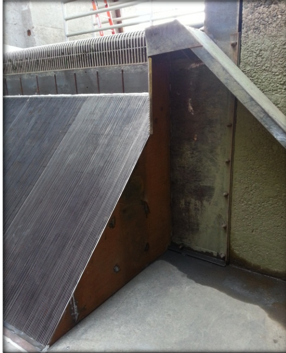
Figure 10 Approach ramp/anti-jump ramp and lamprey ramp (upper right hand corner) installed at the Left Bank Wanapum Fishway Exit Passage System. The approach ramp/anti-jump ramp was installed on June 12, 2014.
