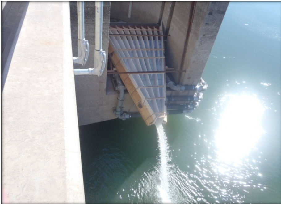
Figure 5 Wanapum Left Bank Fishway Exit Passage System with flume installed.
