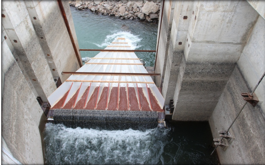
Figure 6 Wanapum Left Bank Fishway Exit Passage System completed and operational on April 15, 2014.
