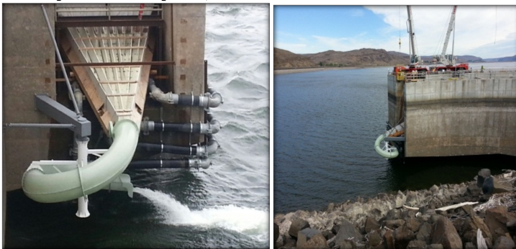
Figure 7 Photograph of installed chutes at the Left Bank and Right Bank Wanapum Fishway Exit Passage System. The spiral chutes were installed on the left and right bank fishway exit passage systems on June 12 and June 19, 2014, respectively.
