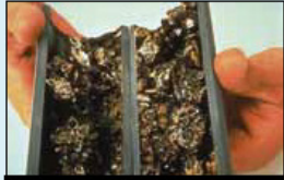
Zebra mussels in a cut-away pipe
